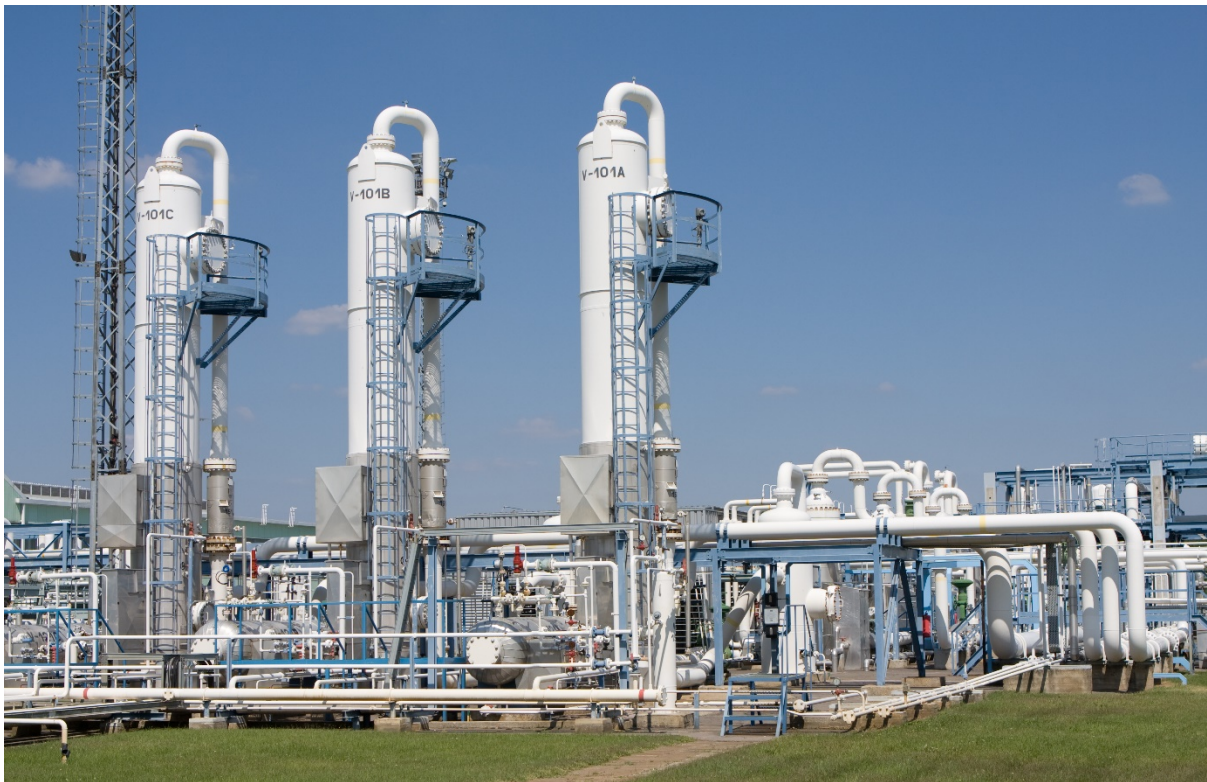
Zsana gas storage facility in Hungary (Hungarian Gas Storage)
